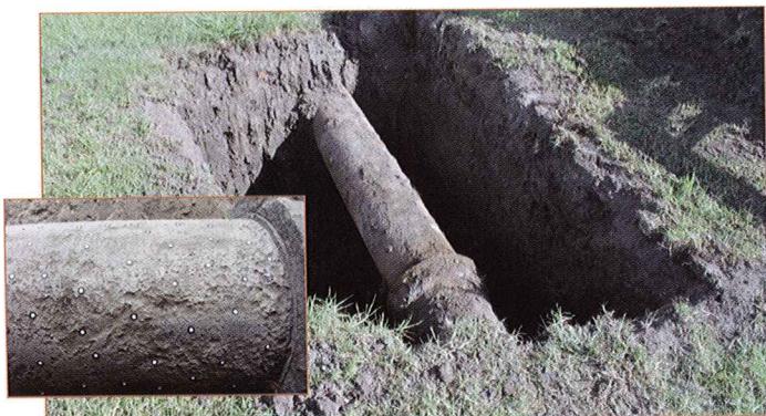
Figure 1: WS4 before abrasive blasting and the sites of maximum corrosion loss after abrasive blasting (inset).
