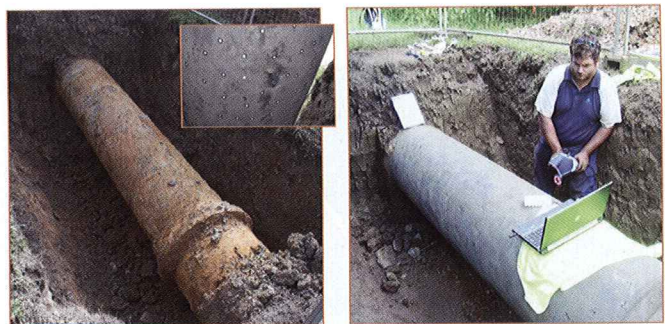
Figure 4: WS5 prior to abrasive blasting (inset – corrosion on bottom of pipe after abrasive blasting).
