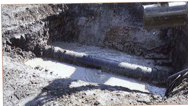
Prediction of failures on underground assets such as this failed DN 500 cast iron pipe are the significant driver of this research.
