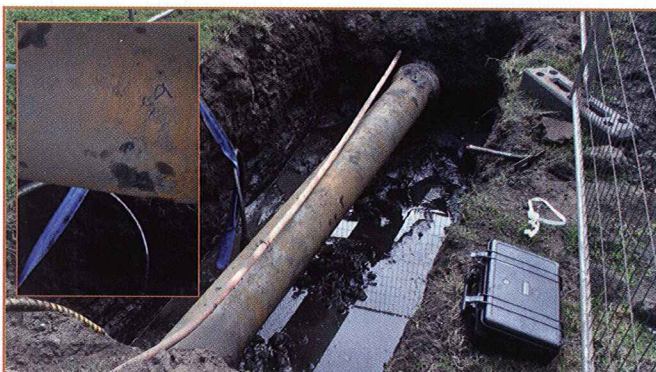
Figure 8: MC4 after abrasive blasting (inset – close up of deepest pit on underside of pipe).
